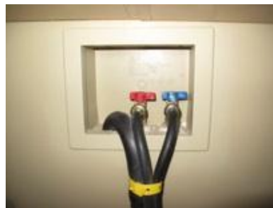
VALVES CLOSED/OFF (handles perpendicular to hoses)
