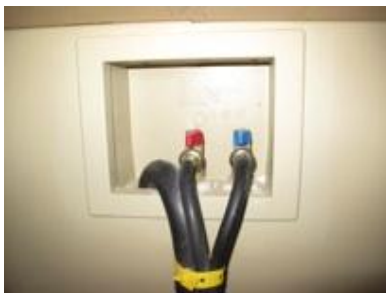
VALVES OPEN/ON (handles in line with hoses) Installed
